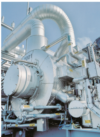
Air conditioning & compressors
