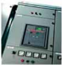
Faults: no problem
